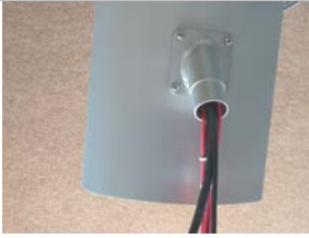
Mast Wiring Exit 014.025
